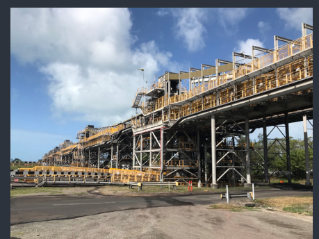
Conveyors & Structural Steel
